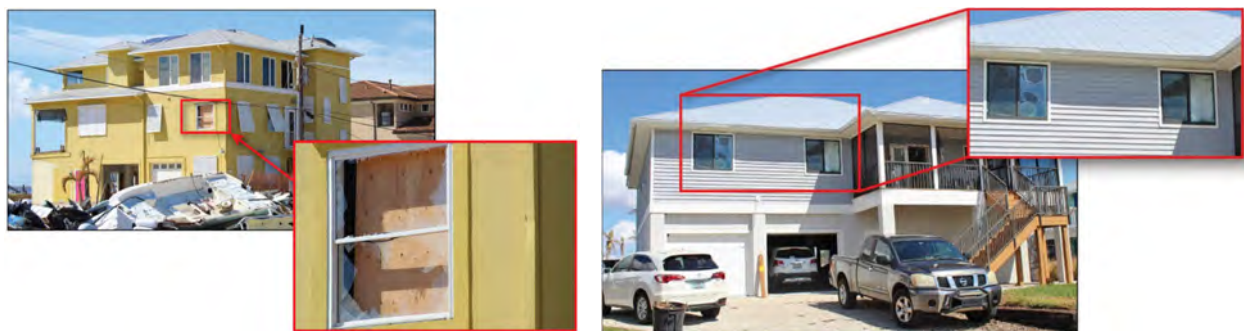
Figure 7. WBD damage to glazing in St. James City (on an inner barrier island in Lee County). The estimated wind speed was 114 mph. (FEMA, 2023)
