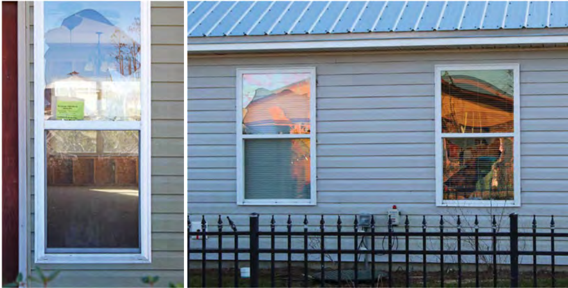
Figure 6. WBD damage to windows in houses in Panama City. The estimated wind speeds were 128 mph (left) and 134 mph (right). (FEMA, 2020)
