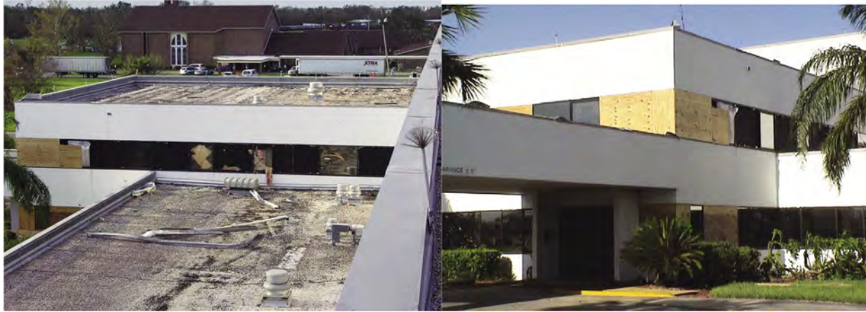
Figure 3. Windows damaged by aggregate at a hospital in Arcadia (inland). Estimated wind speeds between 110-120 mph. (FEMA, 2005)
