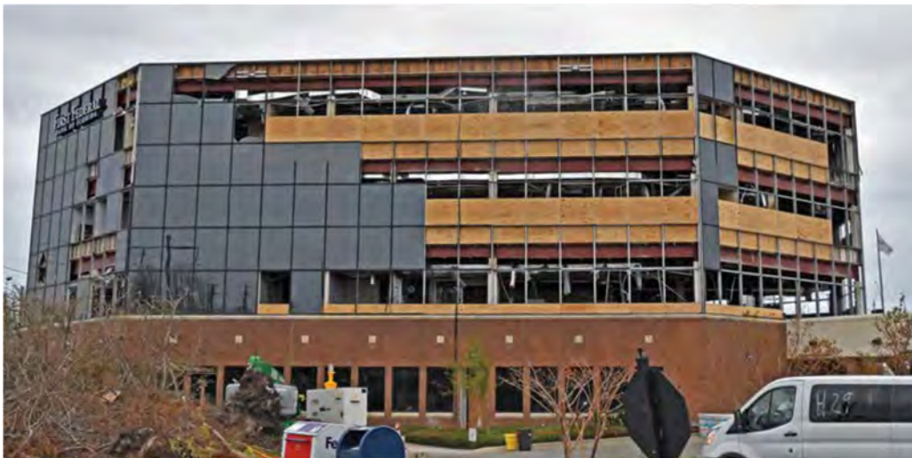
Figure 5. Bank in Panama City with extensive glazing damage. The estimated wind speed was 126 mph. (FEMA 2020).
