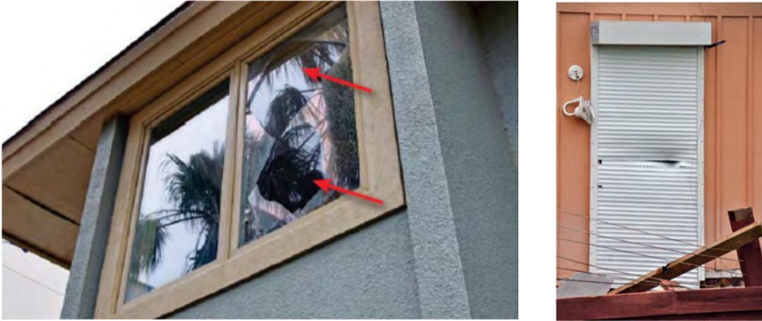
Figure 4. Missile impact damage to roll down shutter, located on an inland bay 10 miles from the coast (left) and glazing damage 5 miles from the coast on inland bay. The estimated wind speed was 120 mph (Exposure C). (FEMA, 2019)
